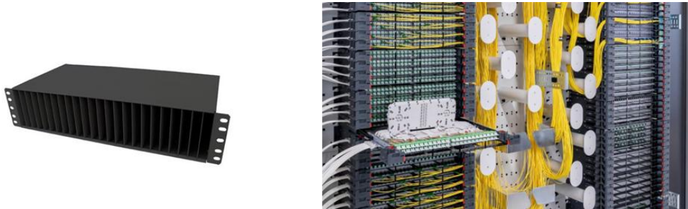
Image. Example of handling of overlength/sling in cable magazines and between racks
